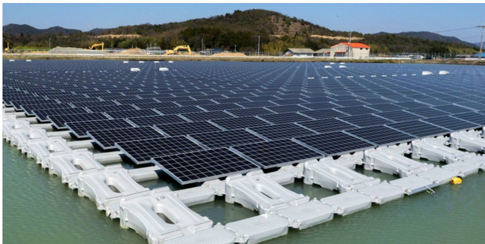
Figure 1.1: Floating Power Plant (FPV)
